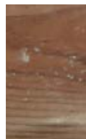
Surface mould/Moho superficial/Moisissures superficielles/Ober- flächlicher Moder/Muf- fa superficiale/Opper- vlakke-schimmel/Bolor superficial
